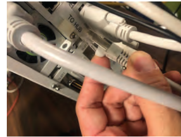
Figure 9 Connect Ethernet Cable to Port 1 on CNS CPU Tower
