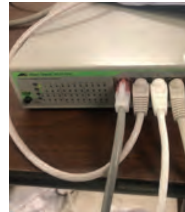
Figure 10 Connected to Ethernet HUB (Network Switch)
